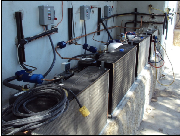
New compressors line the outside wall of the ice plant.
