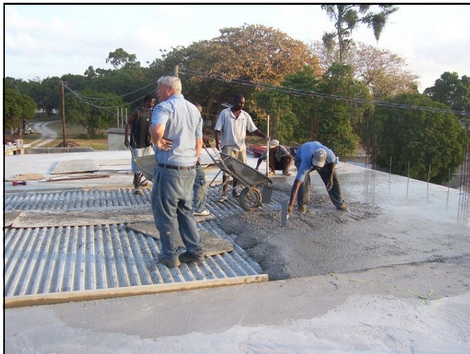
Cement contractor and WISH board member, Fred Hoonhorst from Michigan, directs the pour of the second story floor.
