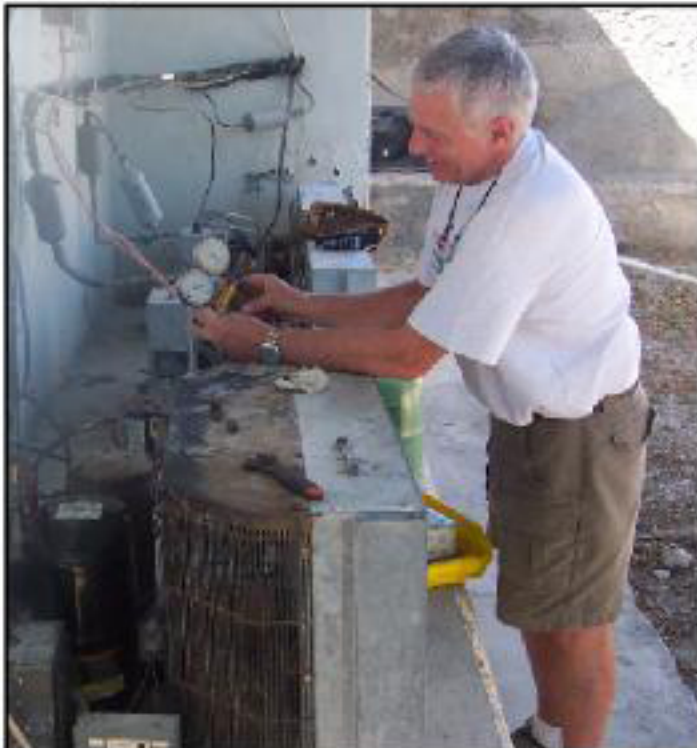
Frank Illingsworth checks gauges on ice plant compressors. Renovations are necessary to increase production.
