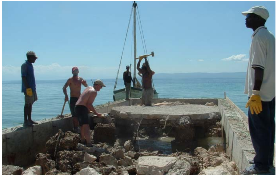
First week of crossings were made in a power boat, all others took about 2 hours in this sailboat. Here the team breaks up the old concrete deck as filler.
