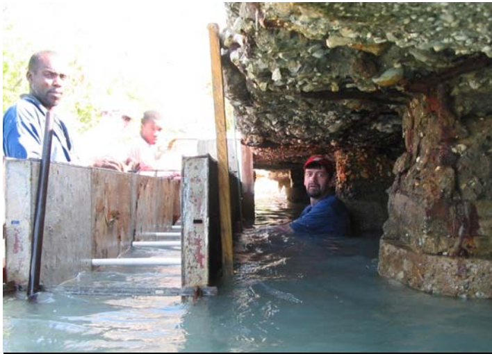
Setting forms required workers to spend many hours working in salt water.
