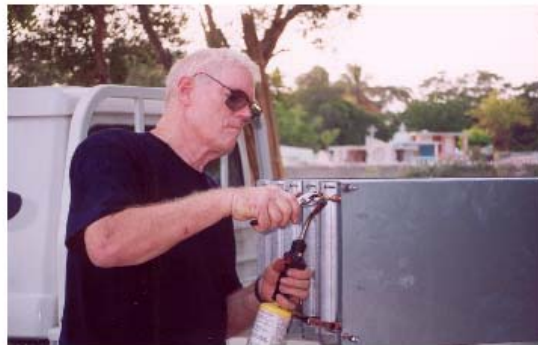
Bob Port solders the freezer plates on an ice machine during his June trip. He plans to return in January to install 2 more machines pending the timely shipment of the container.
